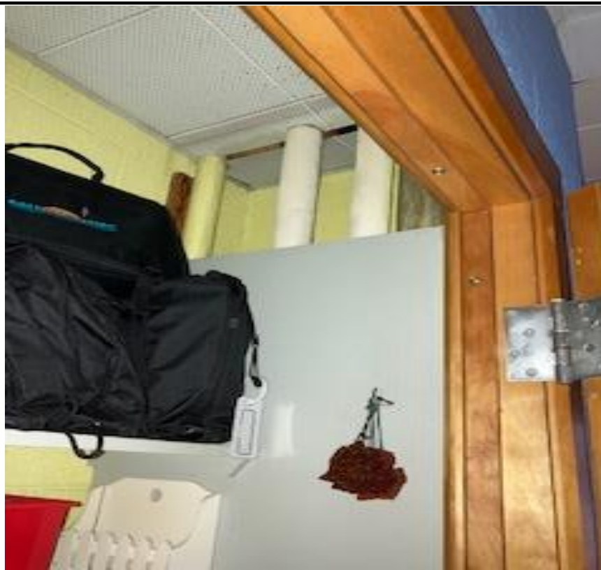
HA#3 Mag insulation riser in office closet
